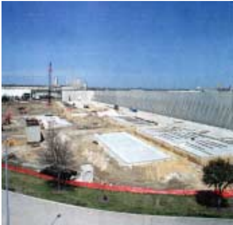
Placement of concrete tilt-wall panels at the Royal Oak Boring Facility in San Antonio, TX
