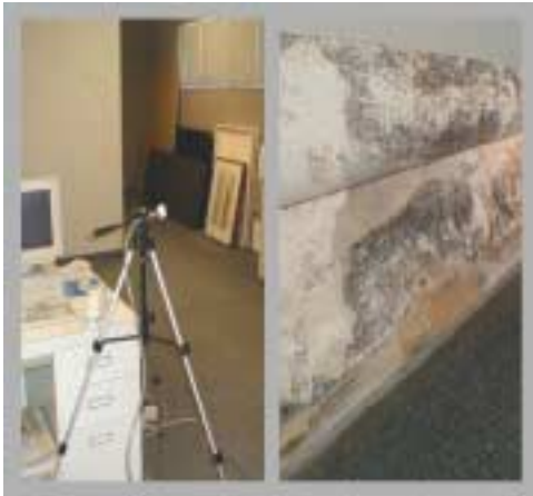
Left: Air Sampling Right: Visible mold proliferation beneath vinyl wallpaper
