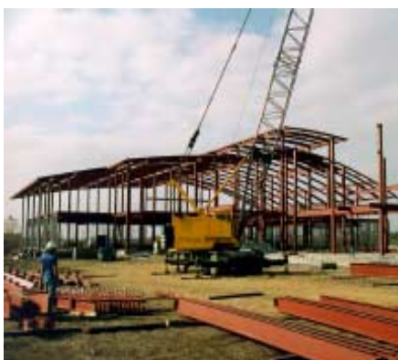
DCE provided construction materials engineering and testing services for the new Palo Alto College Learning Center and Student Center in San Antonio, TX.
