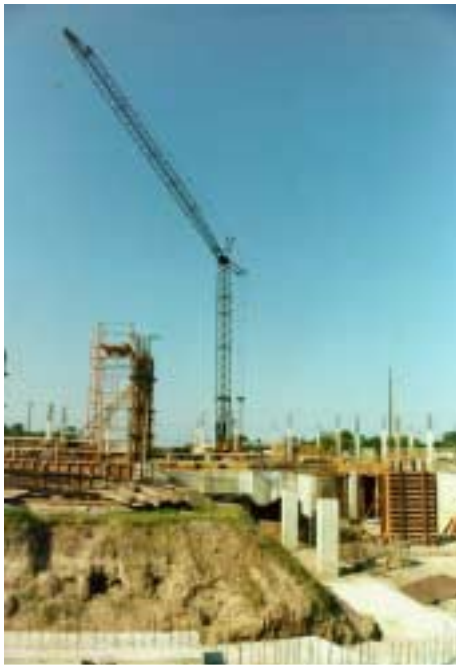
The new U.S. Federal Courthouse and Office Building in Brownsville, TX. DCE provided construction materials engineering and testing services .
