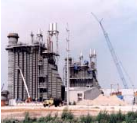
Calpine Power Station, Edinburg, TX
